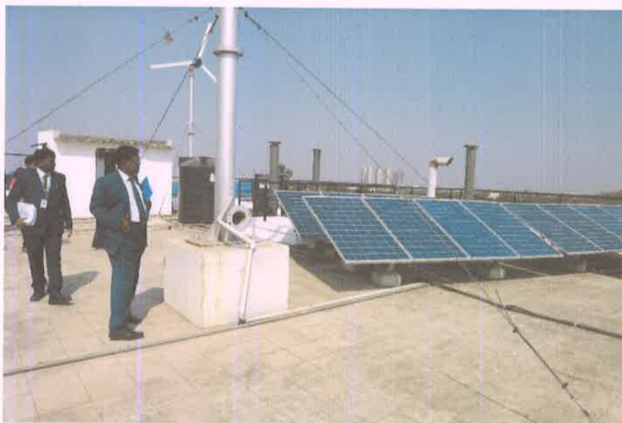
Photograph of Roof Top Solar PV Plant:
