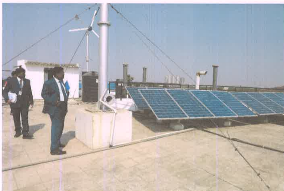
Photograph of Roof Top Solar PV Plant:
