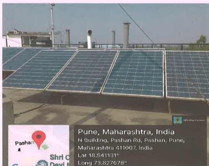
Photograph of Roof Top Solar PV Plant:
