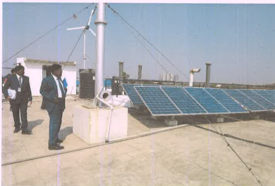
Photograph of Roof Top Solar PV Plant:
