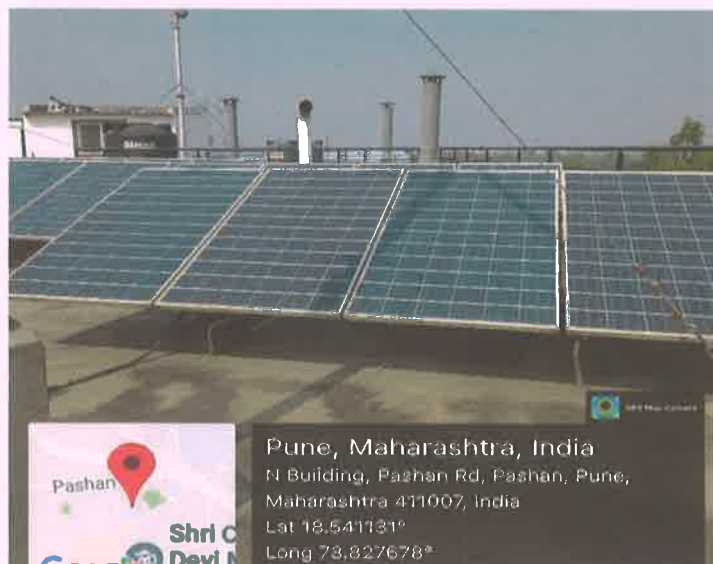
Photograph of Roof Top Solar PV Plant:
