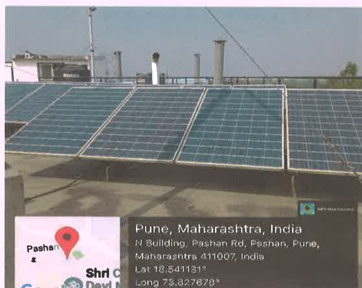
Photograph of Roof Top Solar PV Plant:
